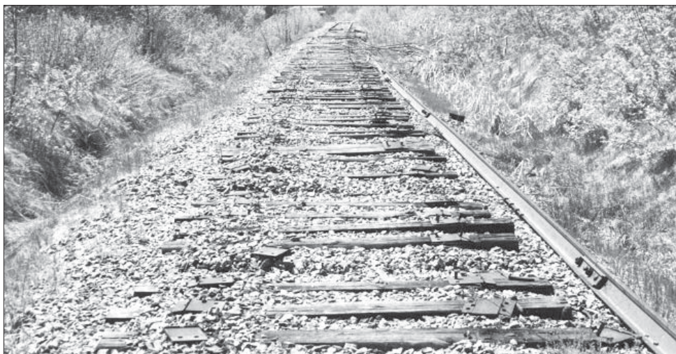
A portion of the Beebe Subdivision railbed shortly before the removal of rails and ties, ca. 1992 (P124 Sentiers Massawippi fonds)
